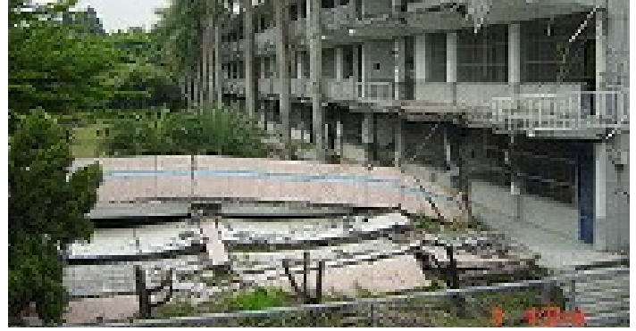
Heavily damaged Guanghu Jr. High School in Wufeng (霧峰區) during the 921 earthquake.
